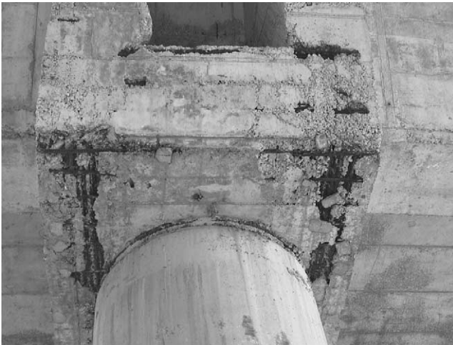
Fig. 2. Typical honeycomb at a column-beam junction.
