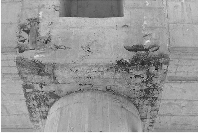
Fig. 10. Steel tying wires at the base of a beam due to non-cleaned forms.
