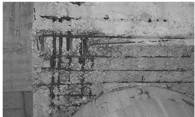
Fig. 9. Steel tying wires at the base of a beam due to non-cleaned forms.
