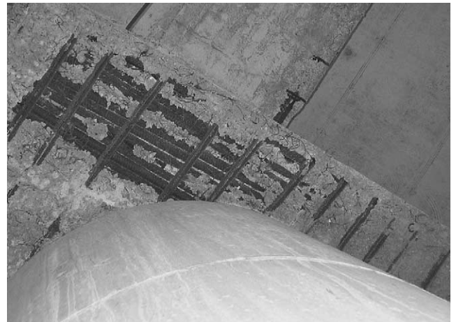
Fig. 5. Reinforcement congestion in a beam.
