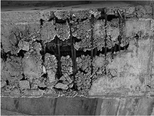
Fig. 1. Typical honeycombs in a reinforced concrete beam.
