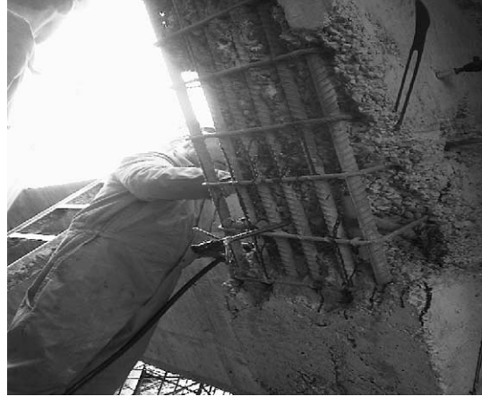
Fig. 8. Clusters of coarse aggregates in a sloped part of a beam.
