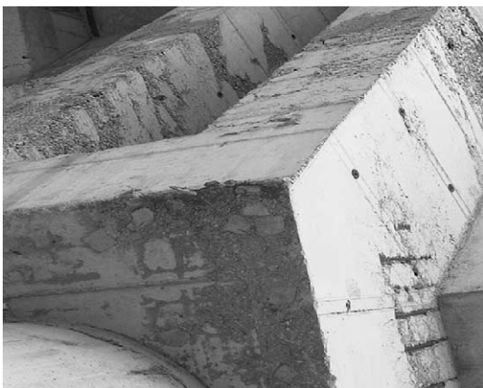
Fig. 7. Clusters of coarse aggregates in a sloped part of a beam.
