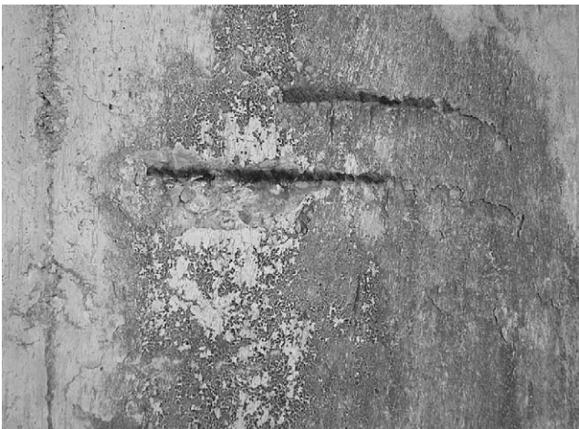
Fig. 3. Steel corrosion at the head of circular column.
