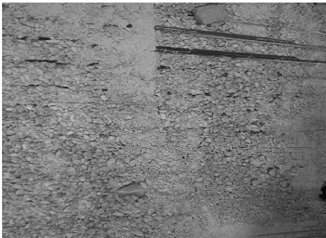
Fig. 6. Clusters of coarse aggregates in a shear wall.
