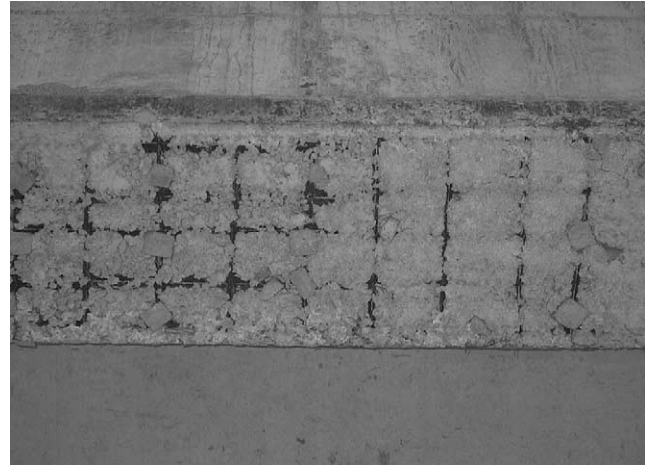
Fig. 4. Inadequate quality of concrete spacers.
