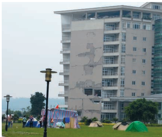
Badly shaken. Students camp outside a damaged SWUST building.
